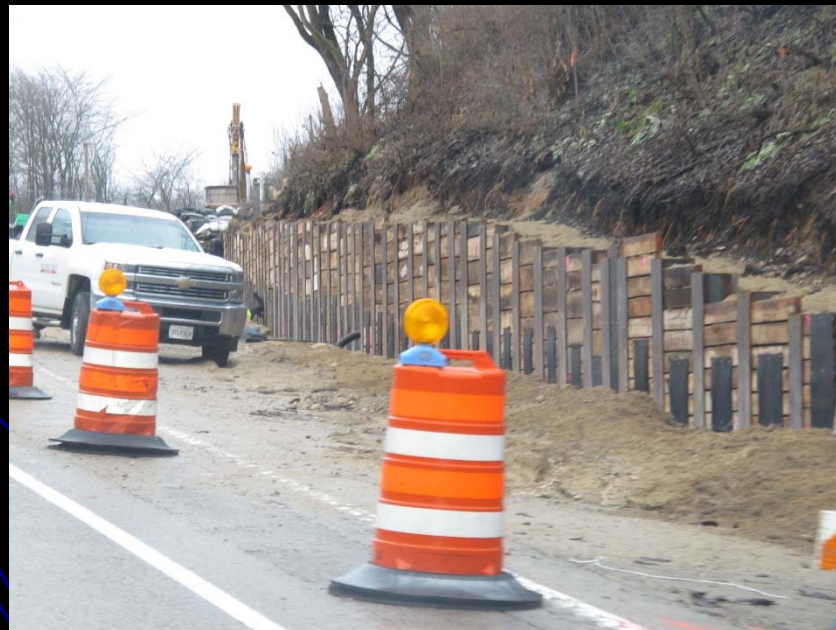
Crews work on lagging for the retaining wall along IL Route 62 as part of the LMP Section D – E/O IL 25 to IL 62 contract
